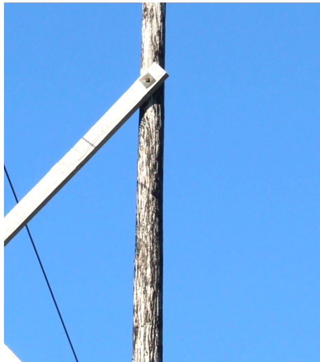
Figure C-8: Deteriorated Pole – Shell Separation
