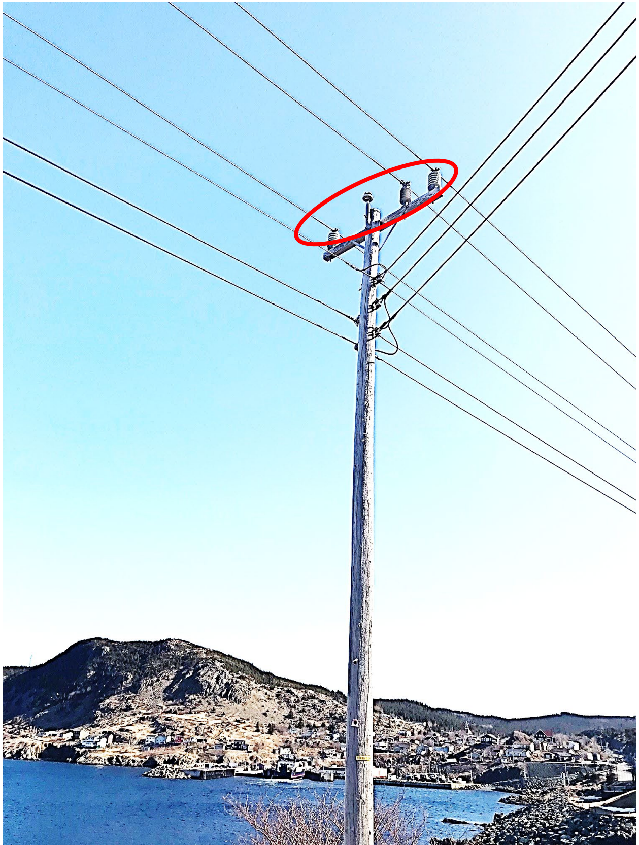
Figure B-2: Insulator Replacement Due to Insulator Flashover
