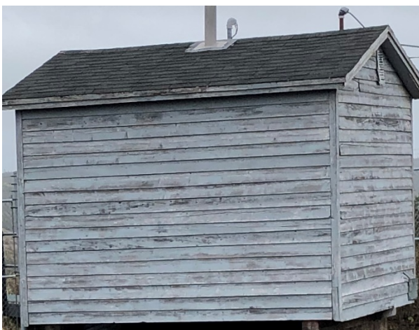
Figure 4: Intake Gatehouse Deterioration
