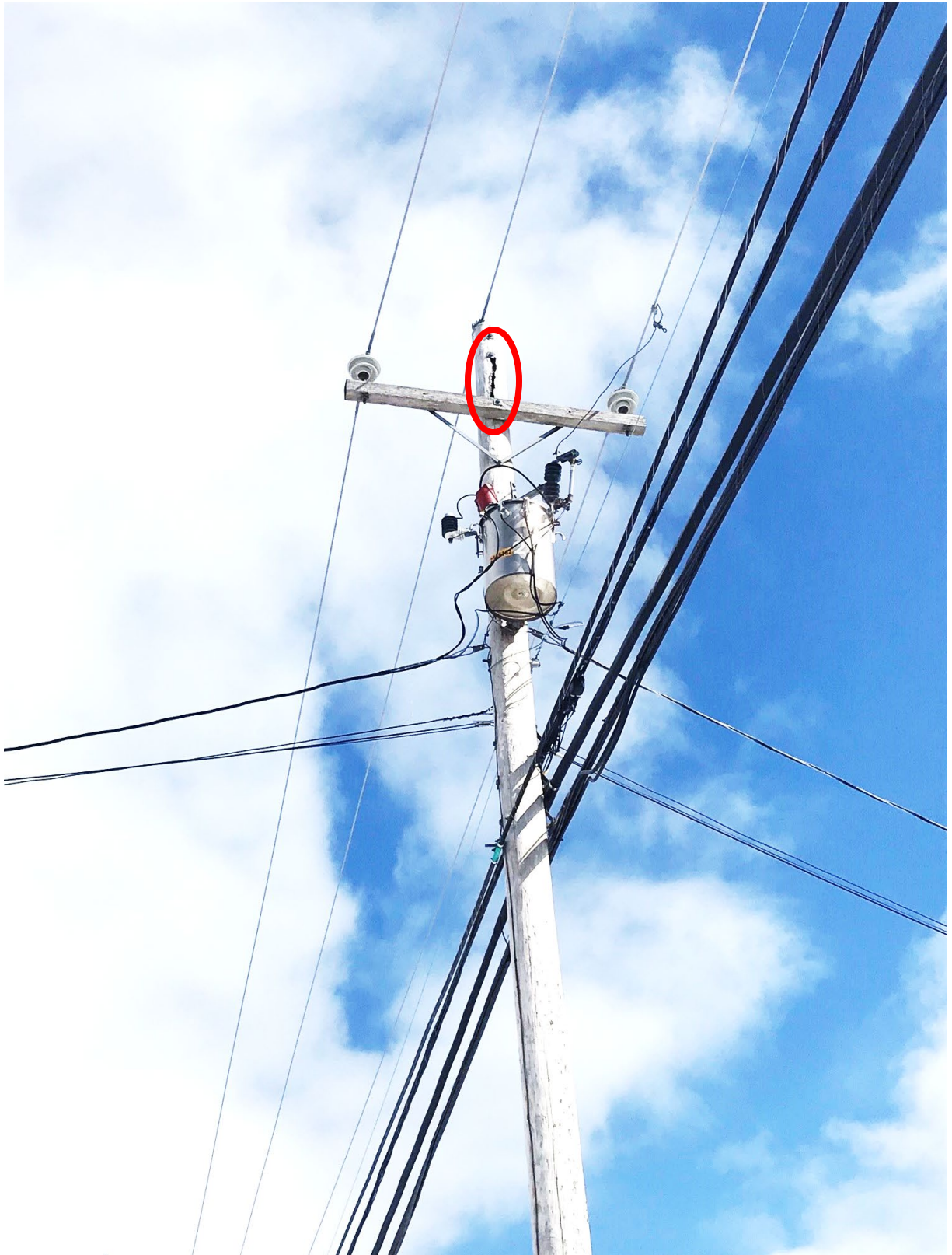
Figure B-5: Insulator Flashover Damage
