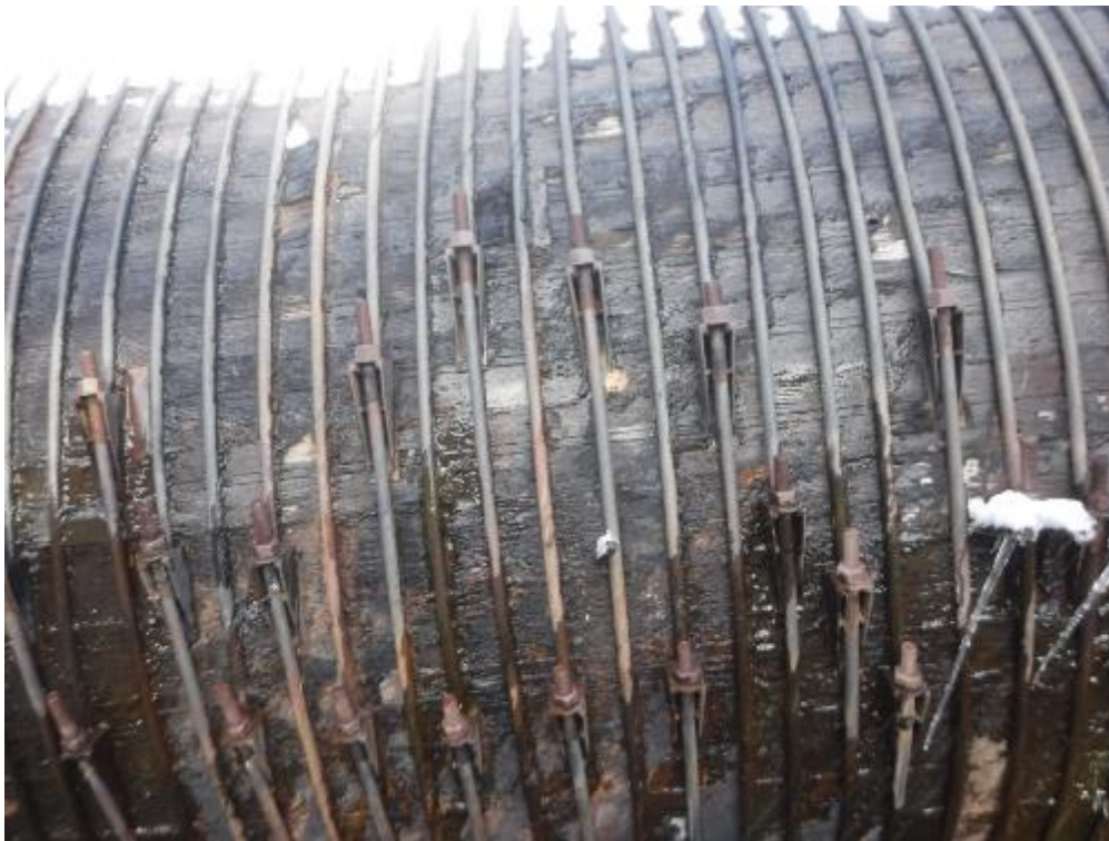
PHOTO 14 TYPICAL BANDS AND WOOD STAVES NEAR POWERHOUSE. SOME CRUSHING AND BROOMING OF WOOD STAVES
