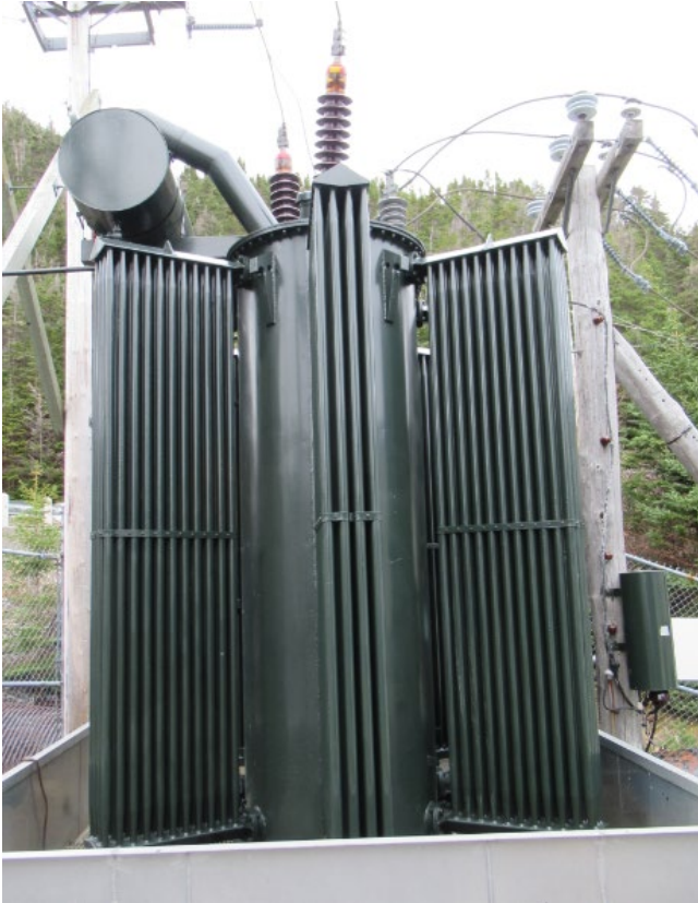
Figure B-3: Tors Cover Substation TCV-T1 Power Transformer
