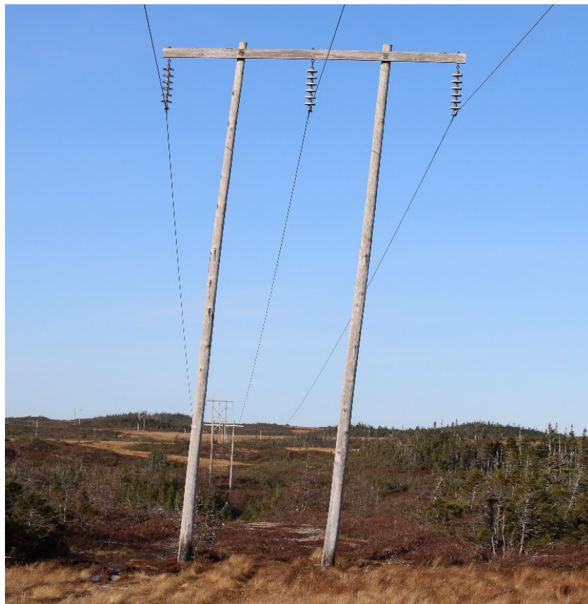
C-16: Leaning Structure – Substandard Construction
