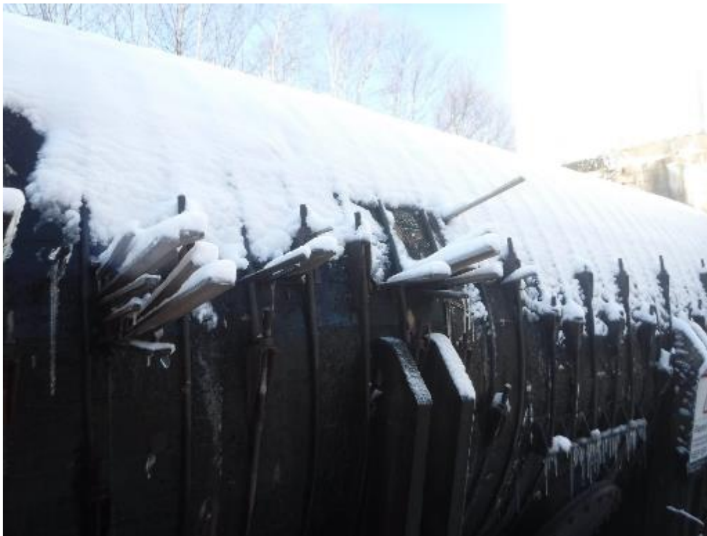
PHOTO 10 SEAM AND SPOT WEDGES DOWNSTREAM OF SURGE TANK
