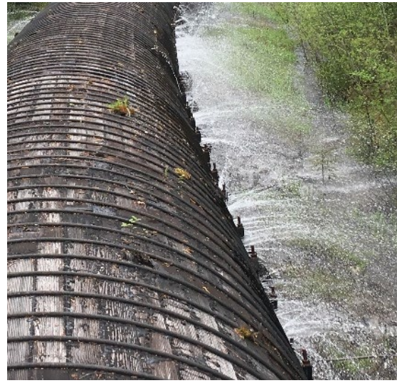
Figure 5: Spring Line Leakage
