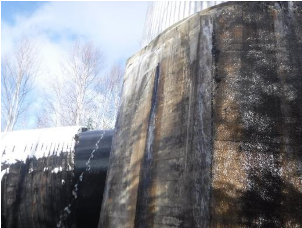
PHOTO 28 WATER POUR FROM CONCRETE FOUNDATION BLOCK
