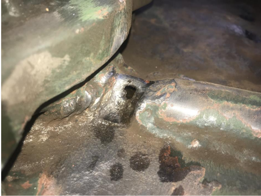
Hole in Transformer Tank Cover near Bushing – Prior to Patch Application
