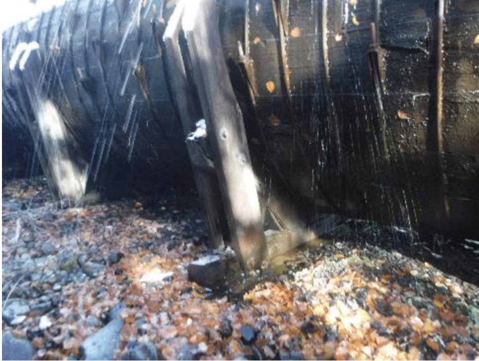
PHOTO 23 SADDLE 36 FROM DAM ON LEFT SIDE – SADDLE IS CRACKED AND LEANING
