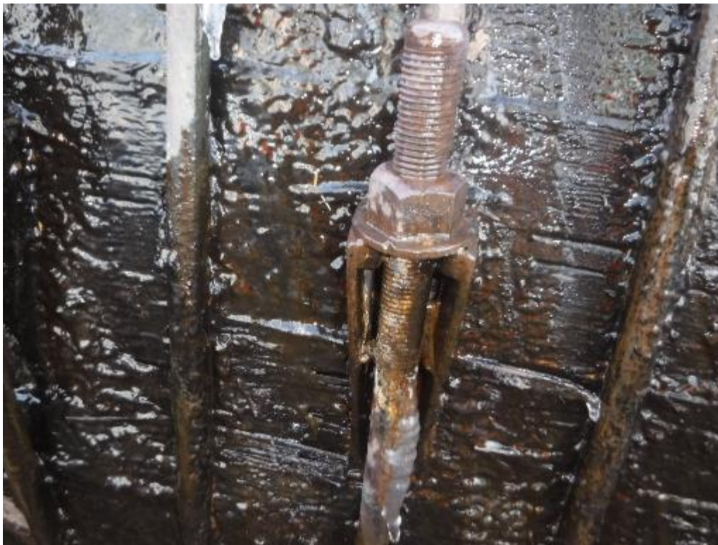
PHOTO 6 TYPICAL BANDING BOLT
