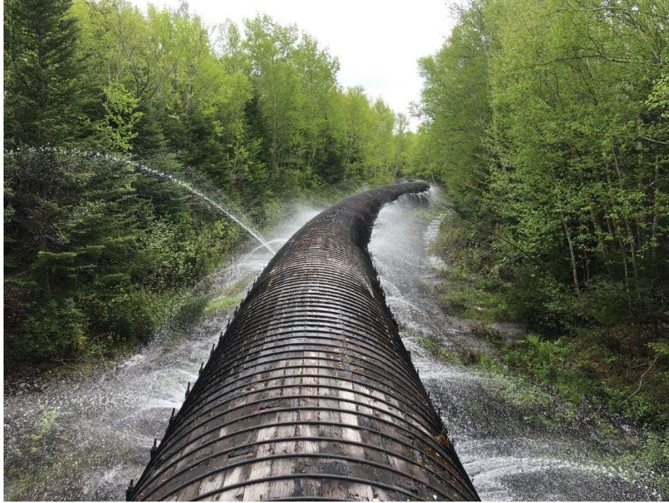
Figure 10: Leakage Along Length of Penstock
