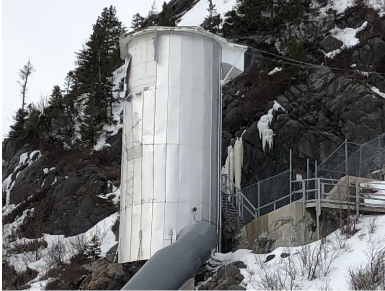
Figure 7: Damage Resulting from “Snowmageddon”
