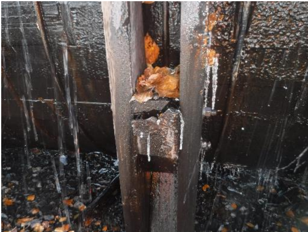
PHOTO 18 SPLIT SADDLE 4 TH DOWNSTREAM OF SURGE TANK ON RIGHT SIDE
