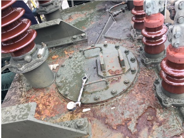
Figure 4: Deterioration on HUM-T2
