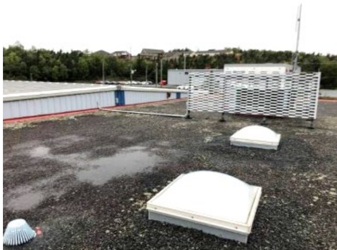
Figure 2: Water Ponding and Displaced Gravel
