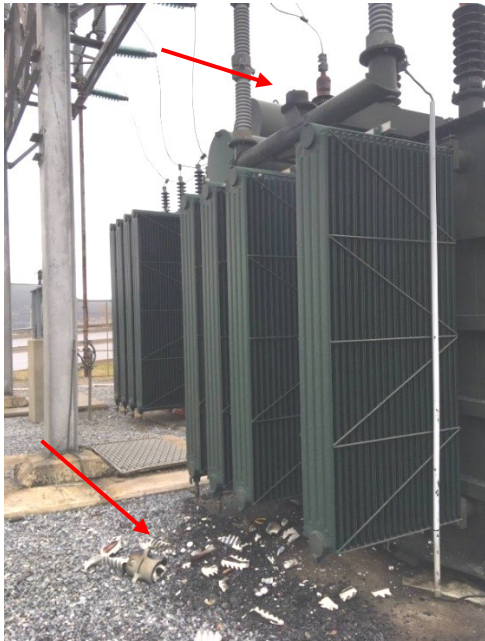
Figure 6: Failed Lightning Arrestor on HUM-T2
