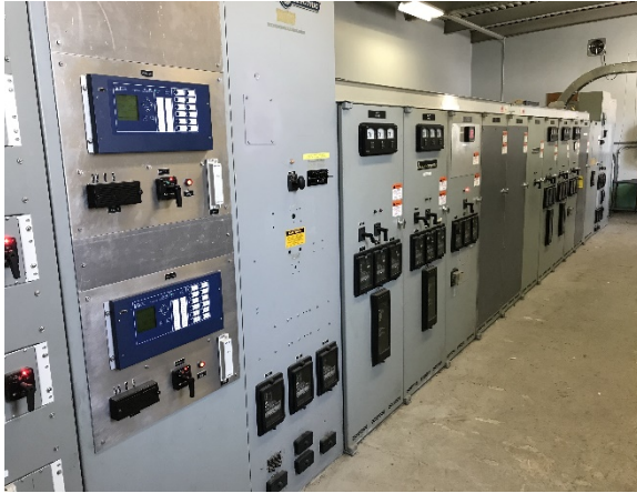
Figure 2: Front Panel of HUM-4.16 kV Switchgear and Substation Controls
