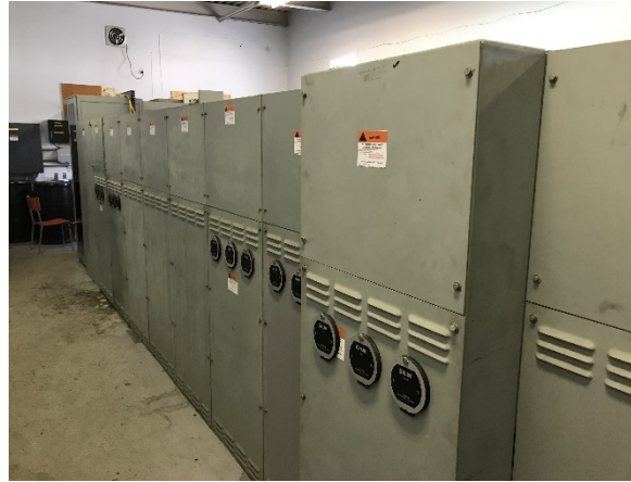
Figure 3: Back of HUM-4.16 kV Switchgear and Substation Controls
