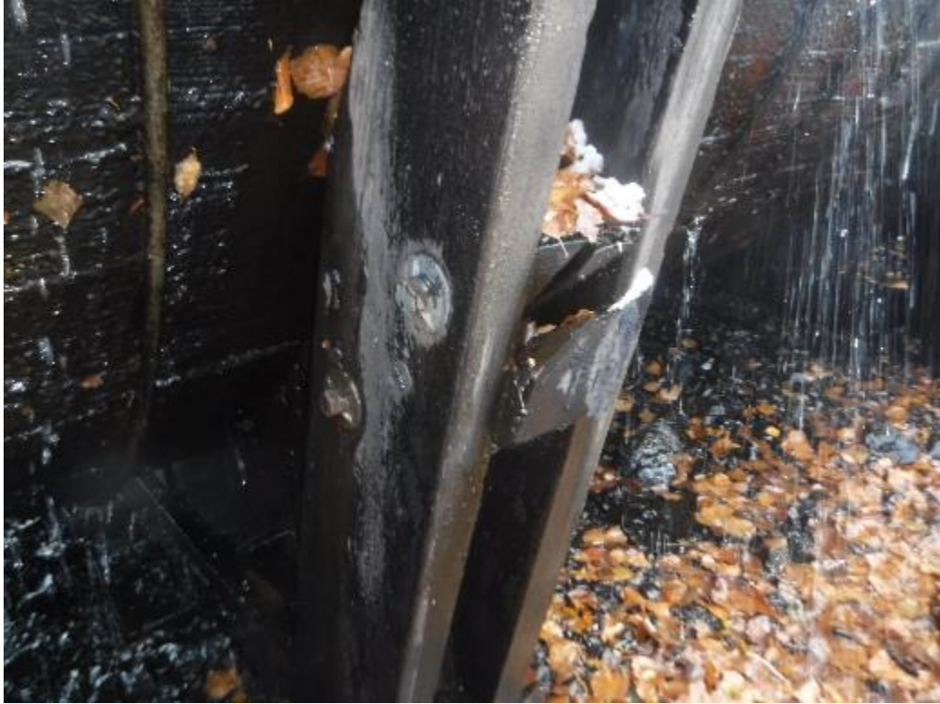
PHOTO 19 SPLIT SADDLE 15 DOWN FROM DAM ON LEFT SIDE. TYPICAL CRACK.
