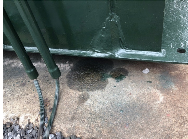
Figure 5: Oil Leak at Previous Repair on HUM-T2
