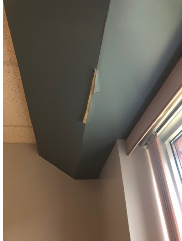
Figure 5: Interior Damage due to Roof Leak
