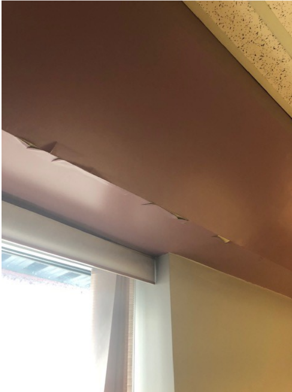
Figure 4: Interior Damage due to Roof Leak
