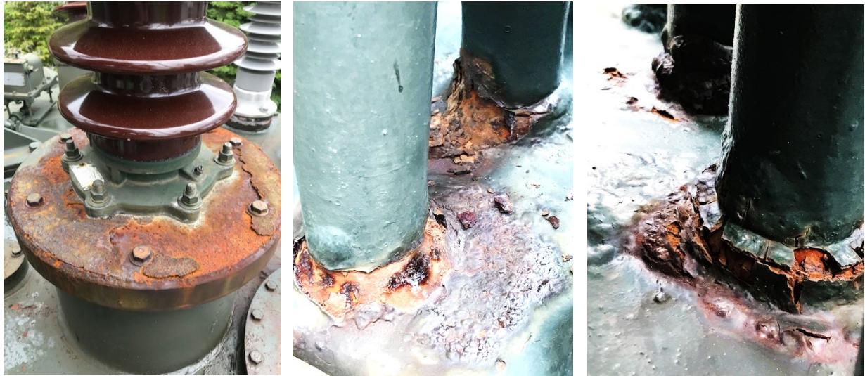
Figure 8: Severe Rust on TCV-T1 Transformer
