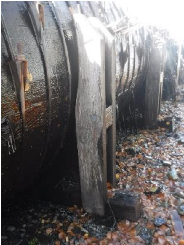
PHOTO 22 SADDLE 100 M UPSTREAM OF SURGE TANK ON RIGHT SIDE. SEPARATION OF SADDLE VERTICAL FROM PENSTOCK
