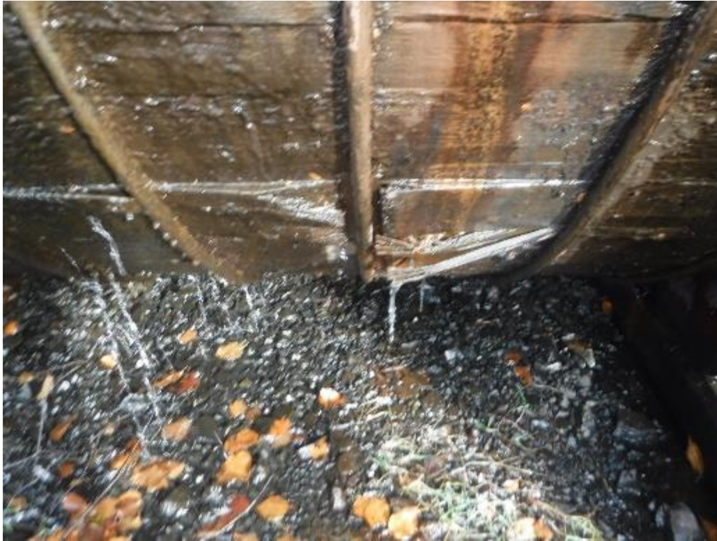
PHOTO 17 BENT AND CRUSHED WOOD NEAR SURGE TANK LEFT SIDE
