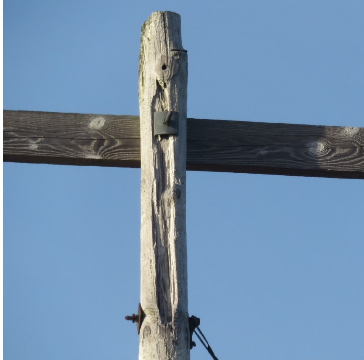
Figure C-7: Deteriorated Pole Top
