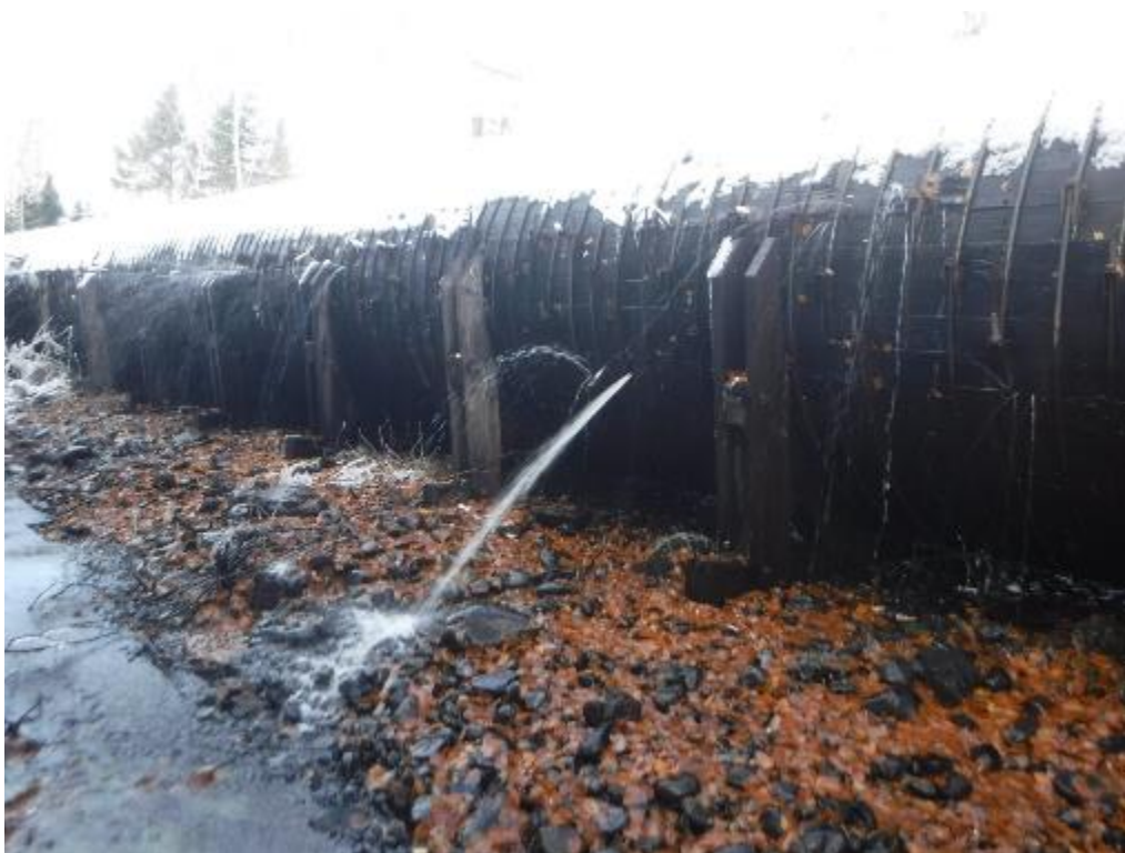
PHOTO 12 WATER JET ON LEFT JUST DOWNSTREAM OF SADDLE 75, NUMBERED FROM DAM
