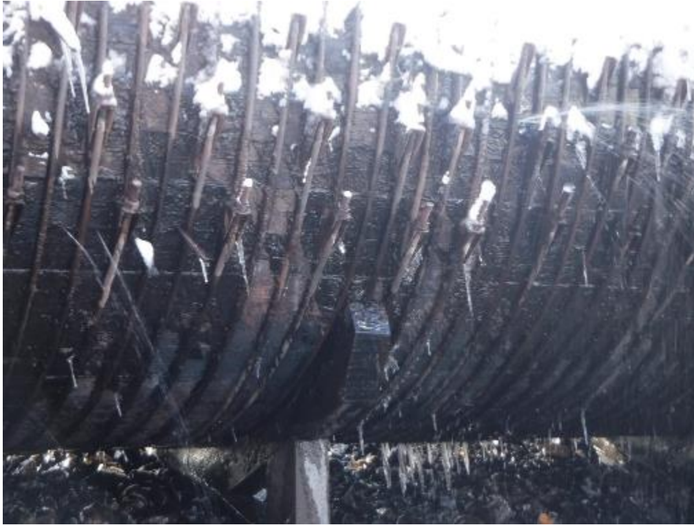
PHOTO 3 TYPICAL BANDING RIGHT SIDE DOWNSTREAM OF SURGE TANK
