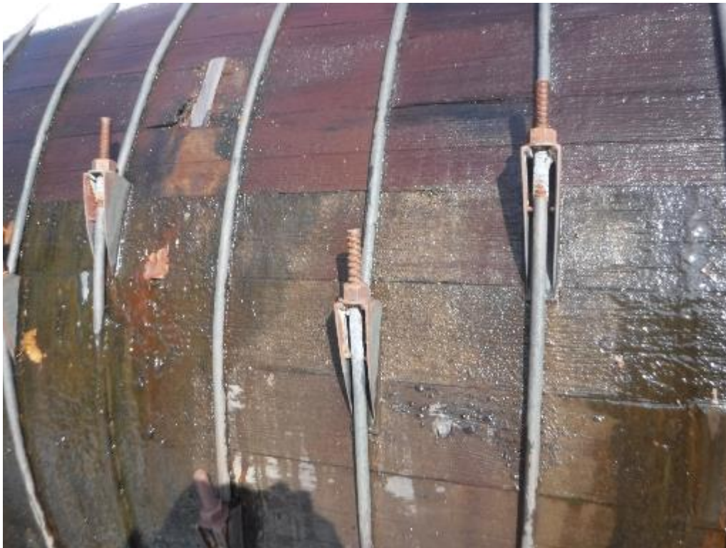
PHOTO 4 TYPICAL BANDING LEFT SIDE UPSTREAM OF SURGE TANK
