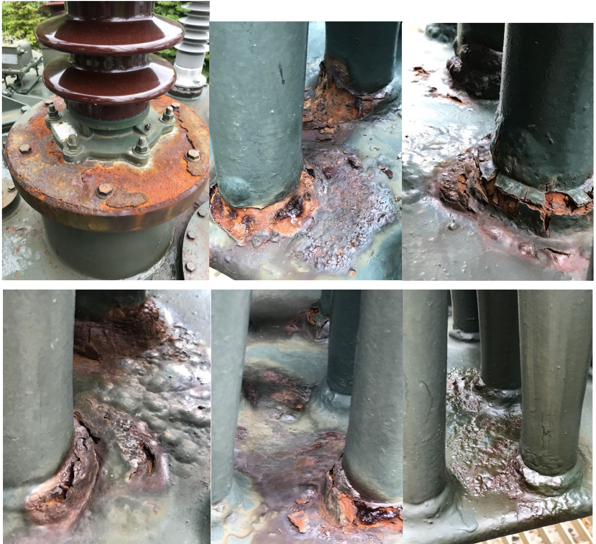
Figure B-4: Tors Cove Substation TCV-T1 Power Transformer – Severe Rusting
