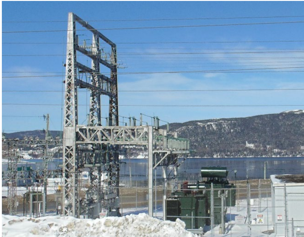
Figure 4: 66 kV Bus Structure, T2 and T3
