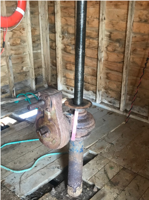
Figure 2: Head Gate Operator
