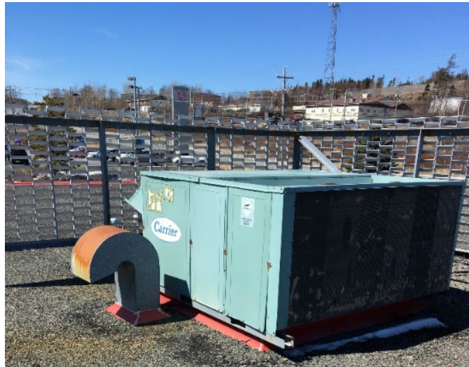
Figure 9: Rooftop HVAC Unit
