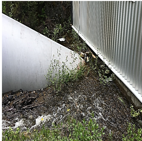
Figure 9: Penstock Entering Powerhouse
