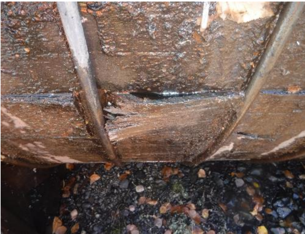
PHOTO 16 CRUSHED AND BROOMING WOOD NEAR SURGE TANK RIGHT SIDE
