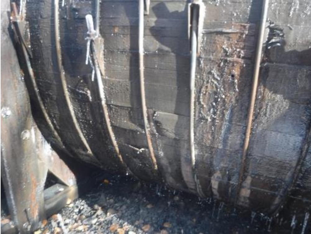
PHOTO 15 BENT AND CRUSHED WOOD NEAR SURGE TANK LEFT SIDE
