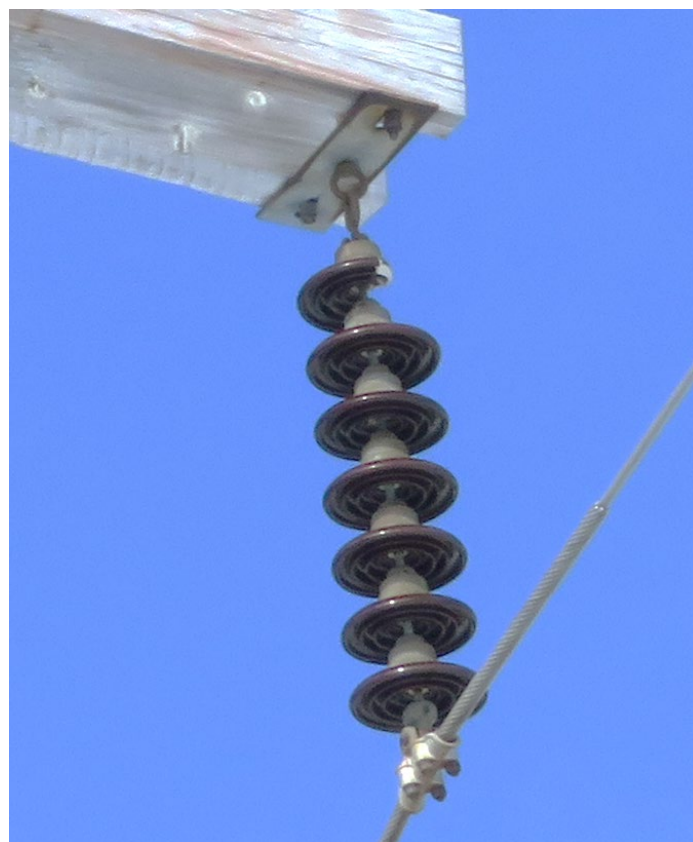
Figure C-6: Broken COB Insulator
