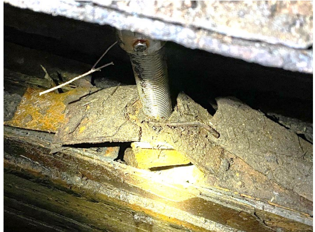
Figure 3: Failed Gate Stem Connection
