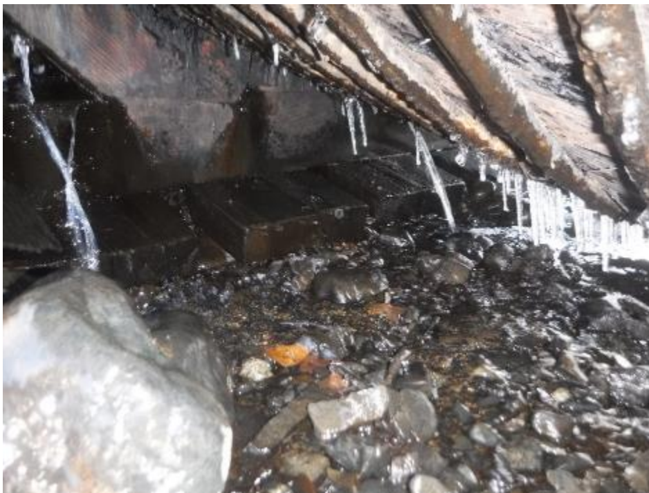
PHOTO 26 SADDLE FOOTING 3 RD UPSTREAM OF POWERHOUSE (TYPICAL CONDITION)
