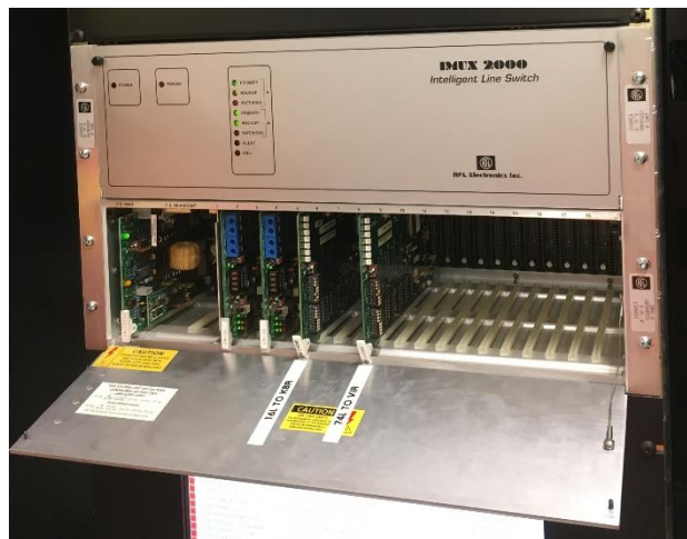
Figure A-4: Typical IMUX Chassis
