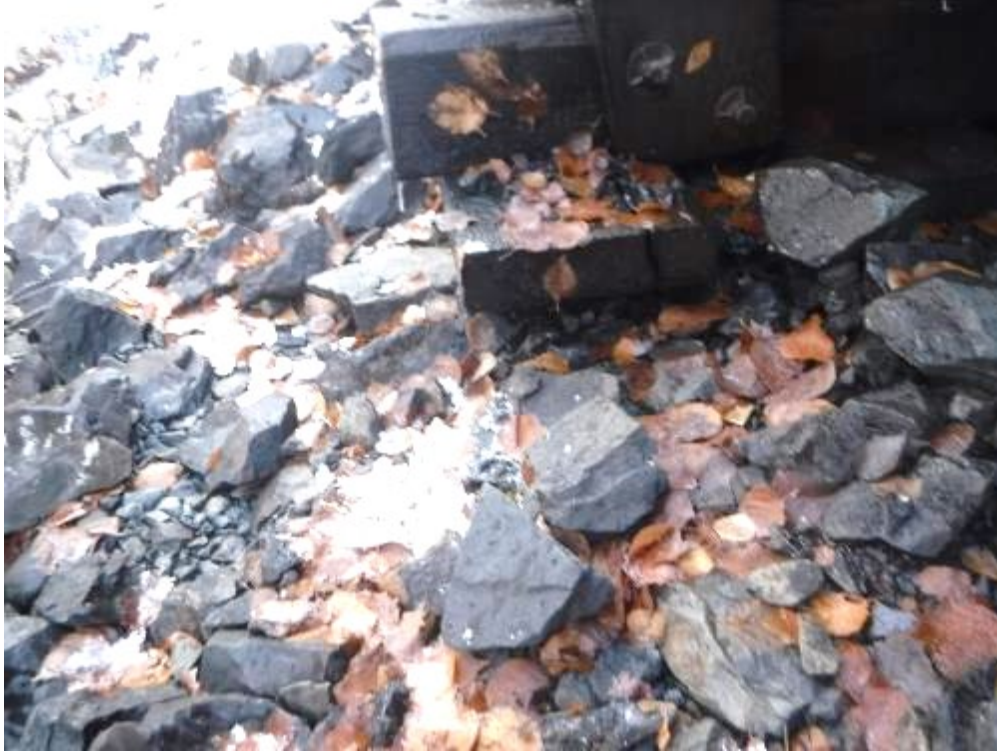
PHOTO 27 SADDLE 27 NUMBERED DOWN FROM DAM ON LEFT SIDE. NOTE FOUNDATION EROSION STARTING
