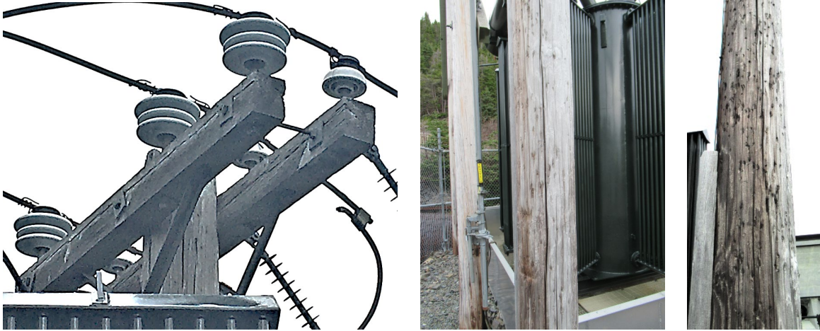
Figure 9: TCV Deteriorated Wood Poles and Cross Arms
