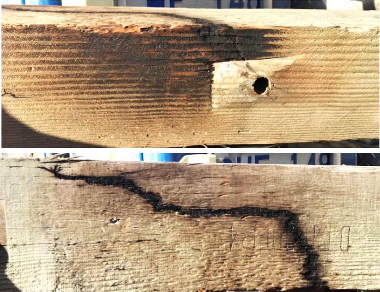
Figure B-6: Evidence of Insulator Flashover on Crossarm
