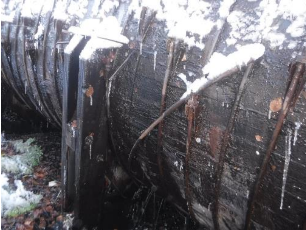
PHOTO 7 DETACHED BAND RIGHT SIDE, ADJACENT 4 TH SADDLE DOWN FROM SURGE TANK
