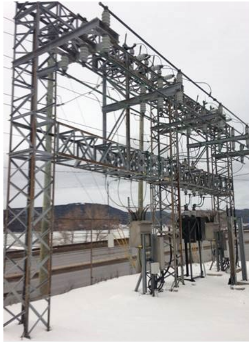
Figure 3: HUM-12.5 kV Low Voltage Distribution Bus Structure
