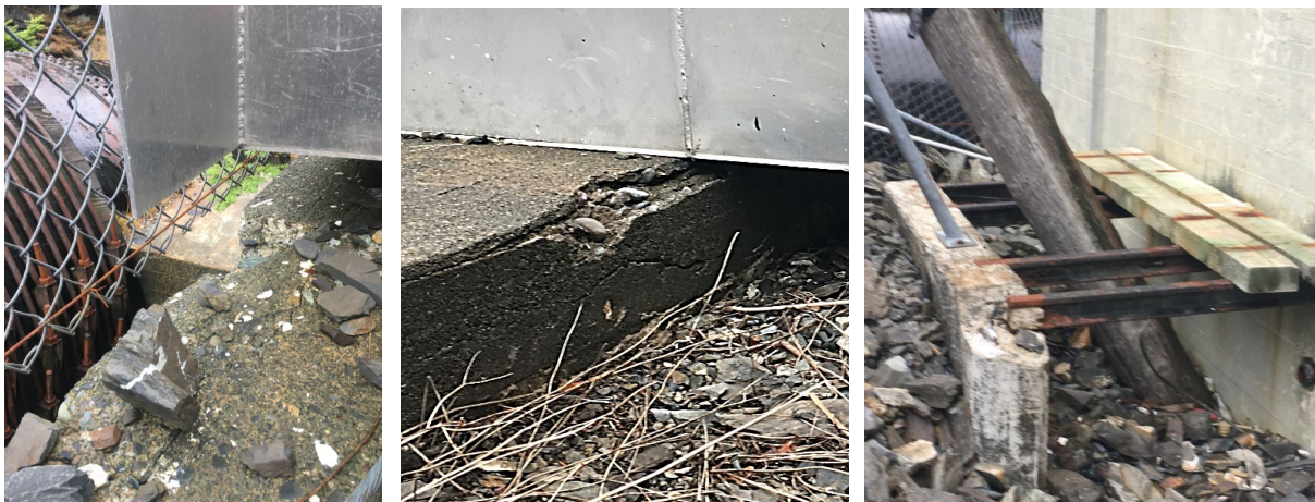
Figure 10: TCV Deteriorated Concrete Foundations
