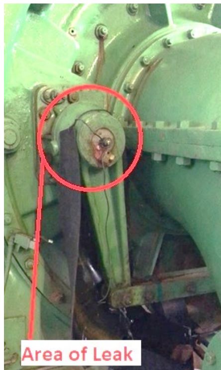
Figure 10: Operating Arm Leakage
