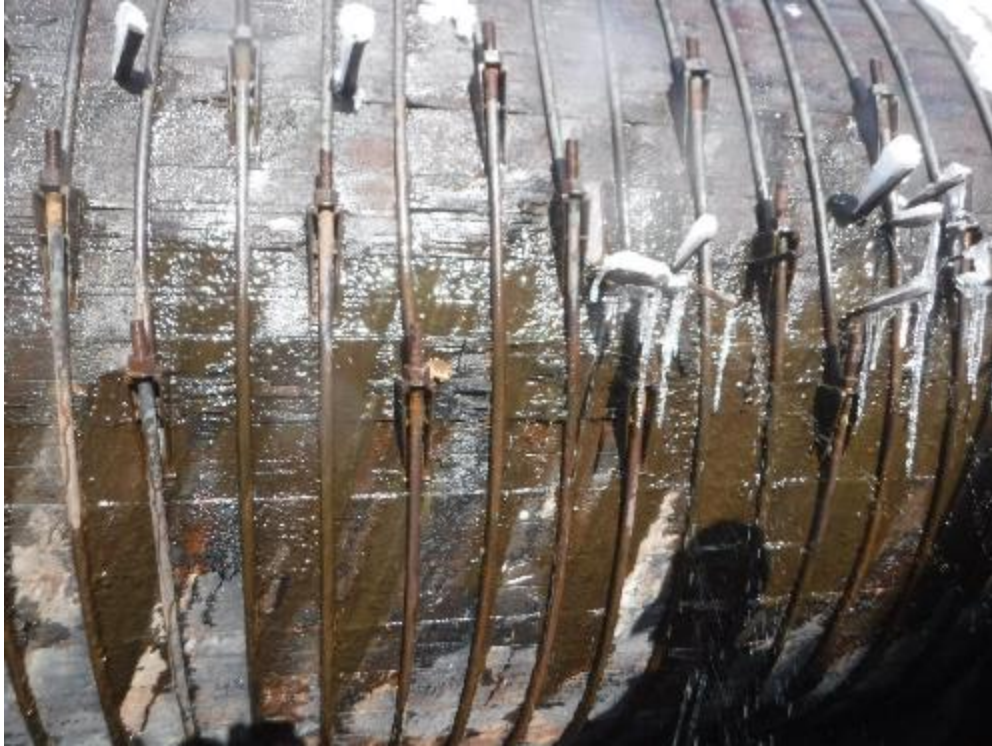
PHOTO 5 TYPICAL BANDING LEFT SIDE DOWNSTREAM OF SURGE TANK
