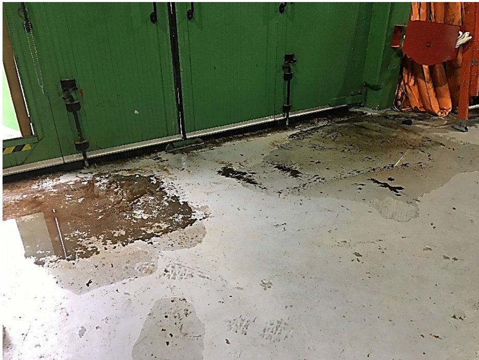
Figure 11: Water in Powerhouse
